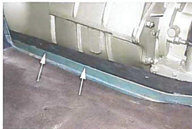
Photo 20: To replicate the original inverted "J" seal, first glue the 1/8 inch thick foam strip to the back side of the metal flange, leaving enough projecting up to reach down to the floor on the front face.
